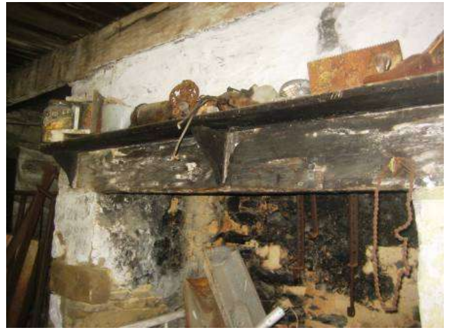
Photo of upper half of the walk-in fireplace in the log cabin.
